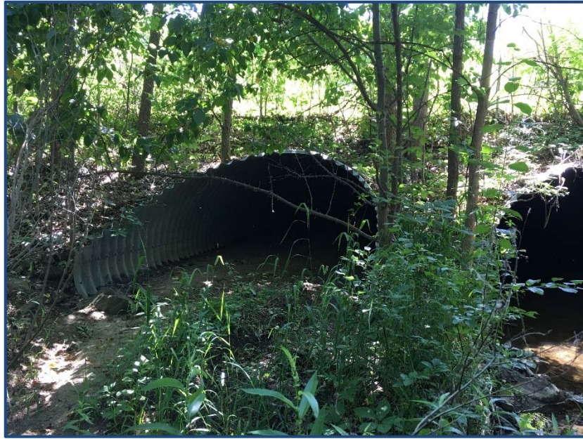
Photo 1. Looking west at existing 7'x10' corrugated metal culverts adjacent to Novi Road, located western edge of the development site (ECT, June 29, 2016).
