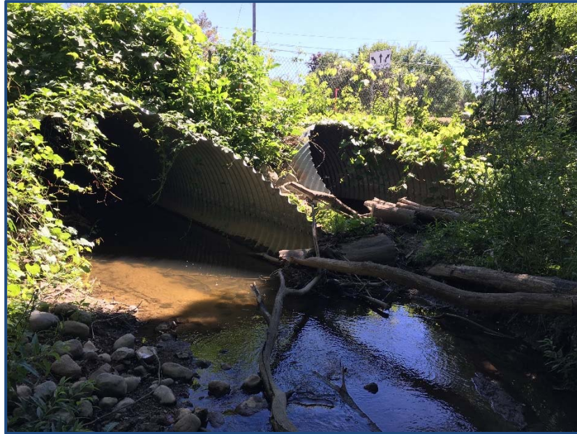
Photo 3. Looking southwest at existing 7'x10' corrugated metal culverts adjacent to Nine Mile Road along the southern edge of the development site (ECT, June 29, 2016).
