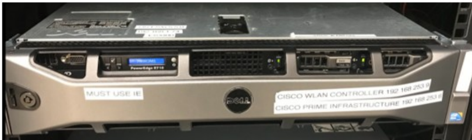
Our old Cisco WLAN Controller (WIFI server) which will be replaced by Meraki cloud technology.
