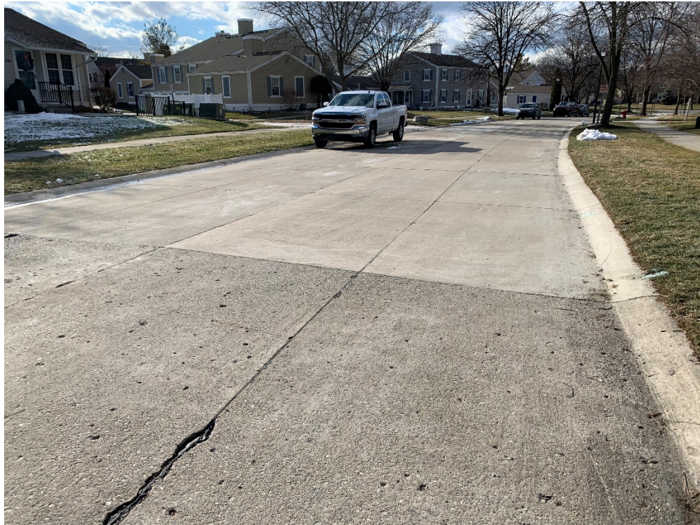
Onaway Drive (Country Place Condominiums) – Full width panel replacements
