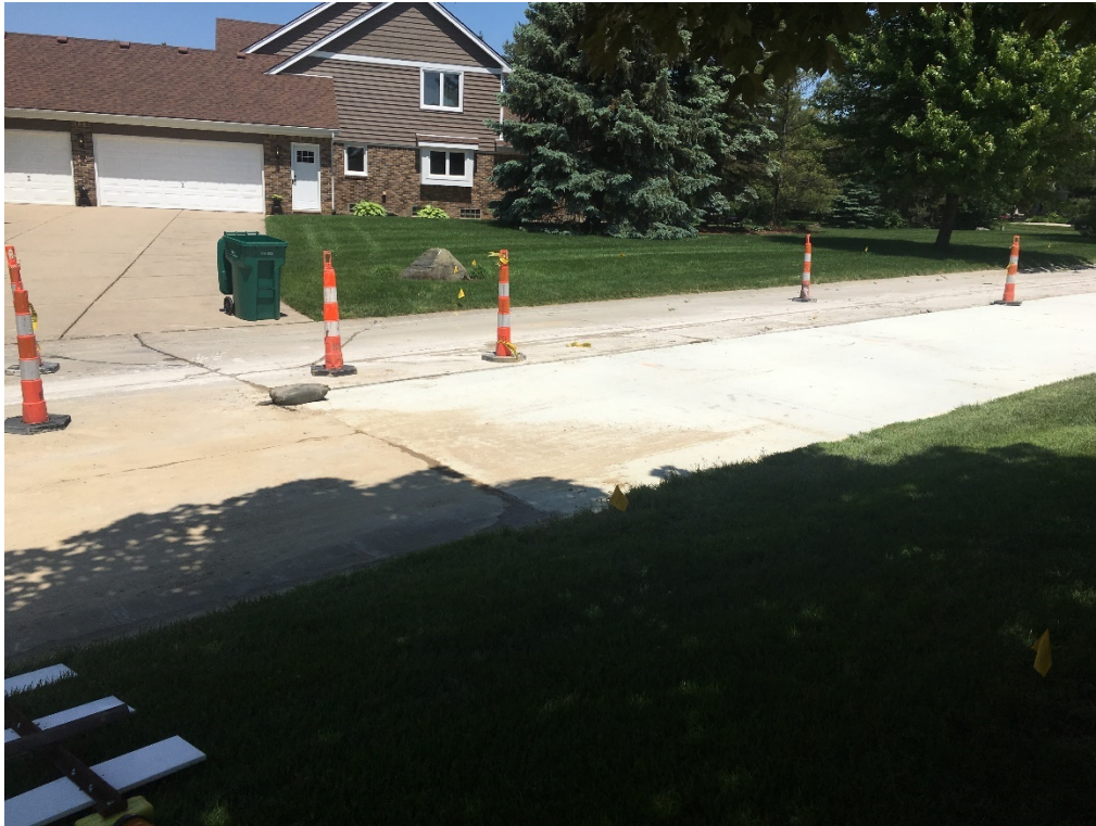
Roxbury Drive (Lexington Green Sub) – Completion of concrete pour for first half
