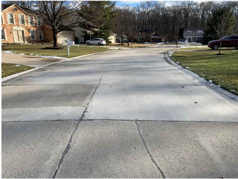
Clover Lane (Whispering Meadows Sub) @ Shadybrook – Intermixed panel replacements
