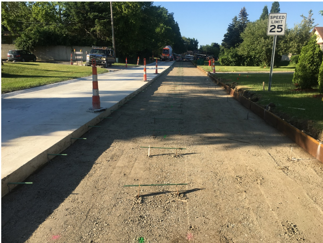
Nilan Drive (Fairfield Farms Sub) @ 10 Mile – Beginning to pour the second side
