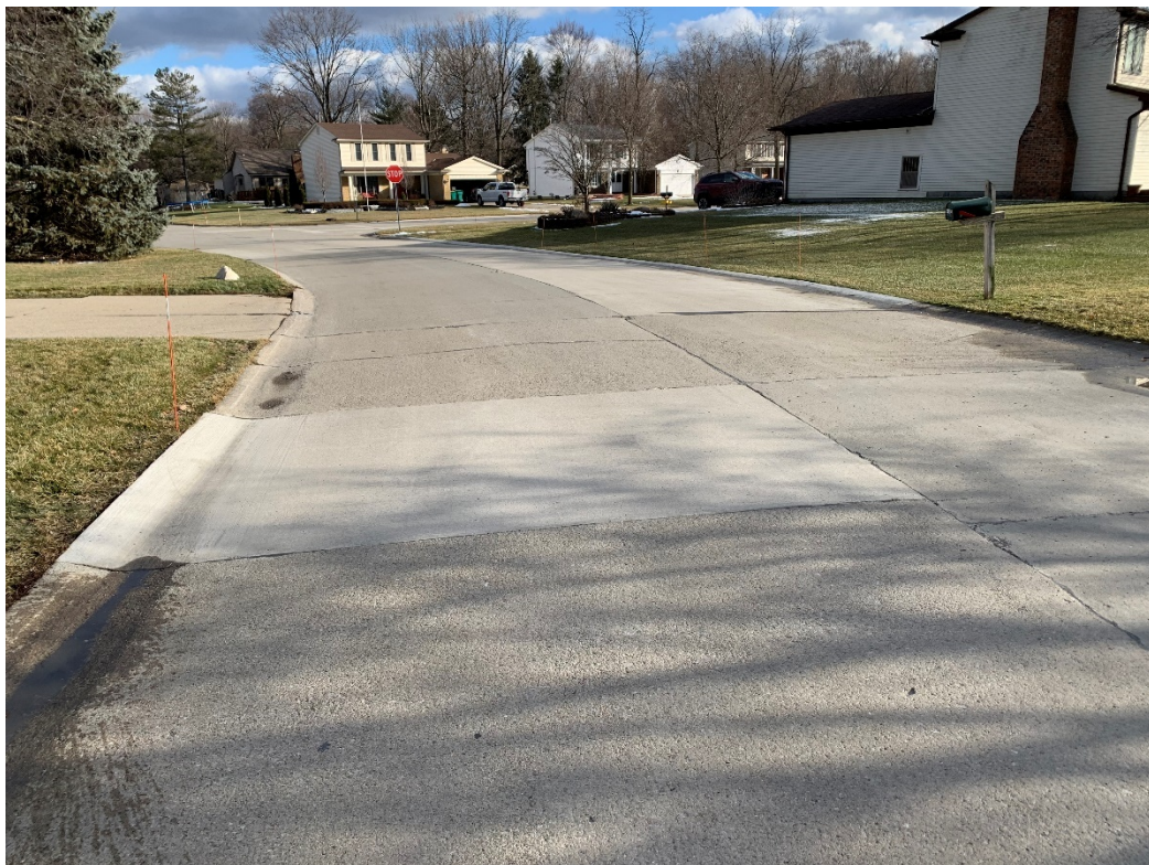
Ladene Lane (Whispering Meadows Sub) – Large panel replacements
