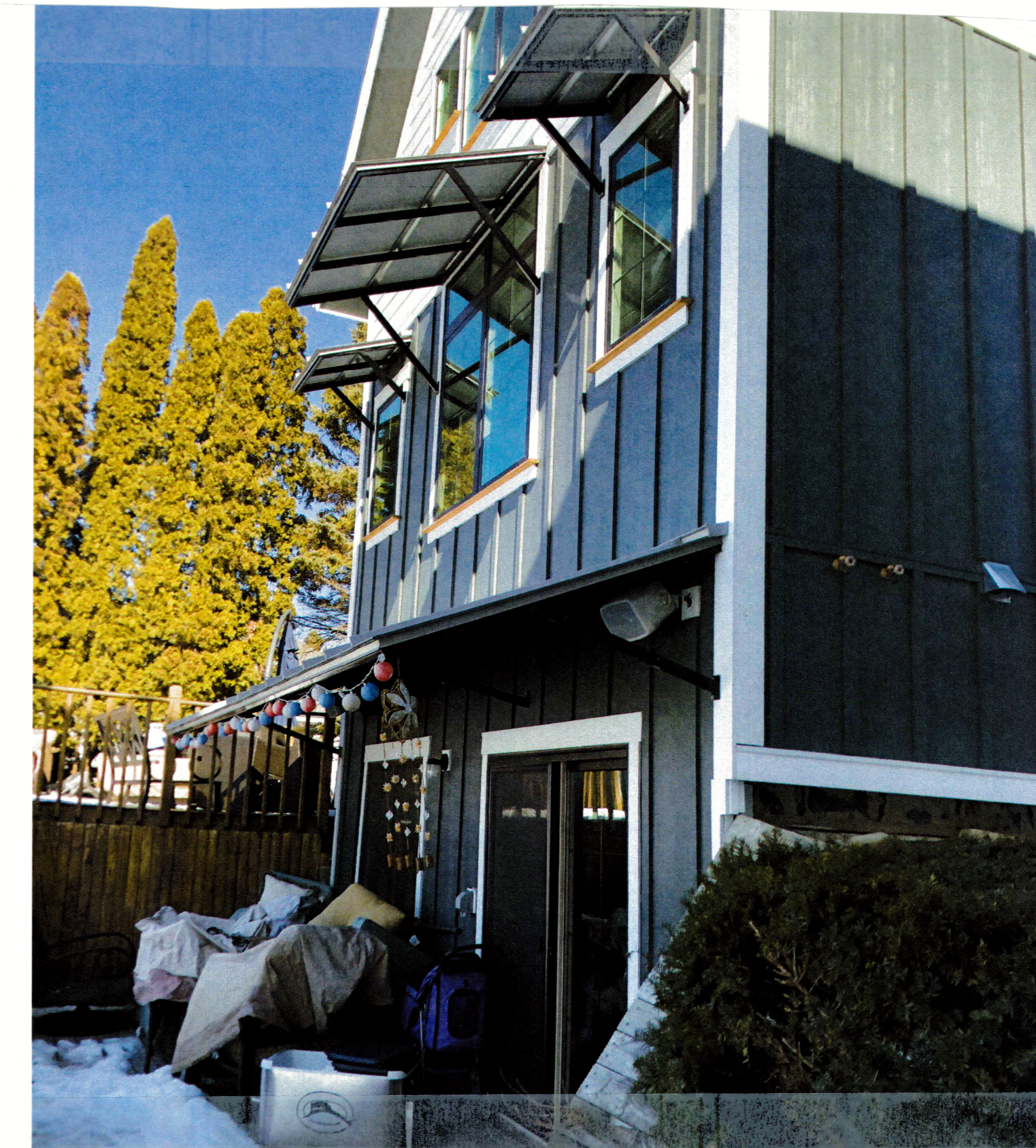
View of existing lake front elevation with first floor elevation below the existing grades on each side.
