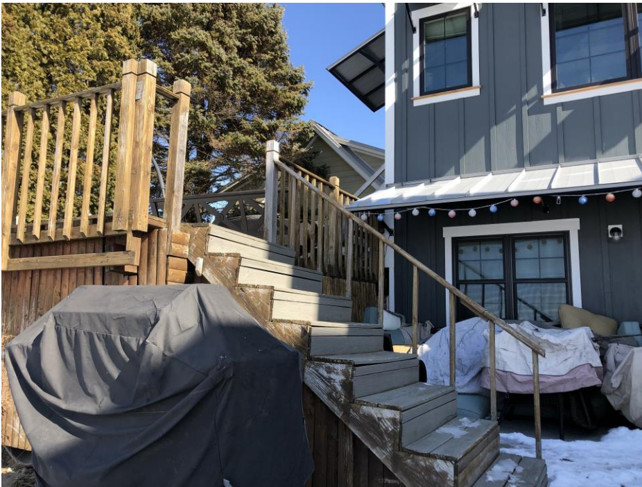
LAKE-FRONT VIEW FROM FIRST FLOOR OBSCURED BY PRE-EXISTING WOOD DECK & STAIRS IN DISREPAIR.
