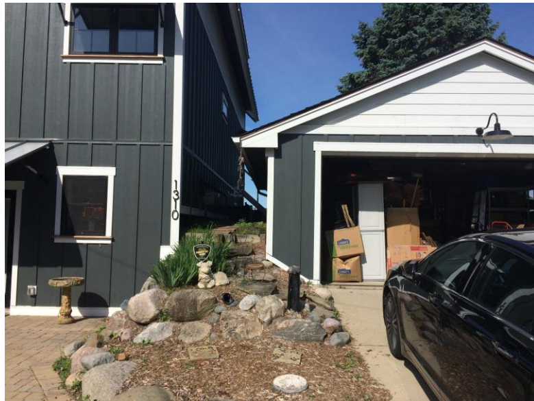
POOR ACCESSIBILITY OF HOUSE CONNECTION TO THE DETACHED GARAGE The garage floor is 30" above the house floor line with man door on opposite side of the garage.
