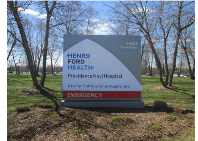
Existing 9'-0" x 11'-0" signage to be removed & replaced; Install far enough away to avoid existing footer
