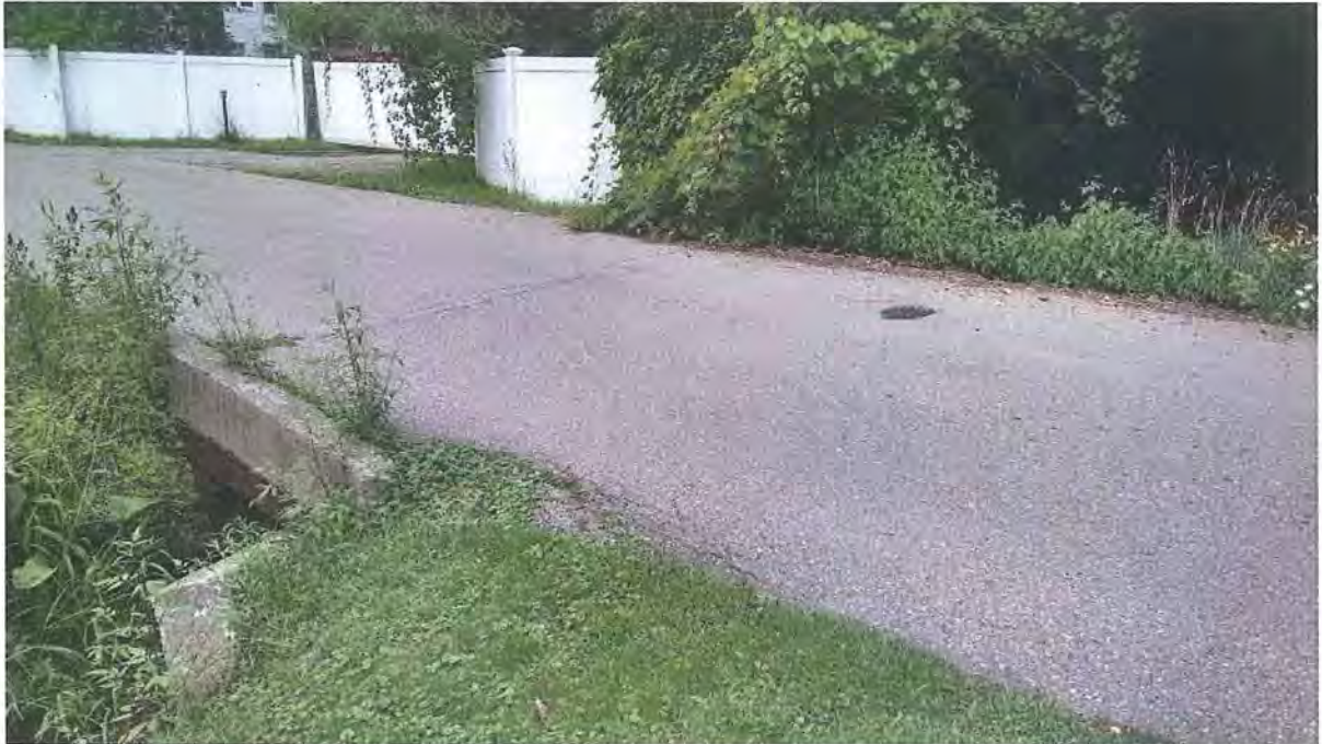
Sink Hole Recently Observed
