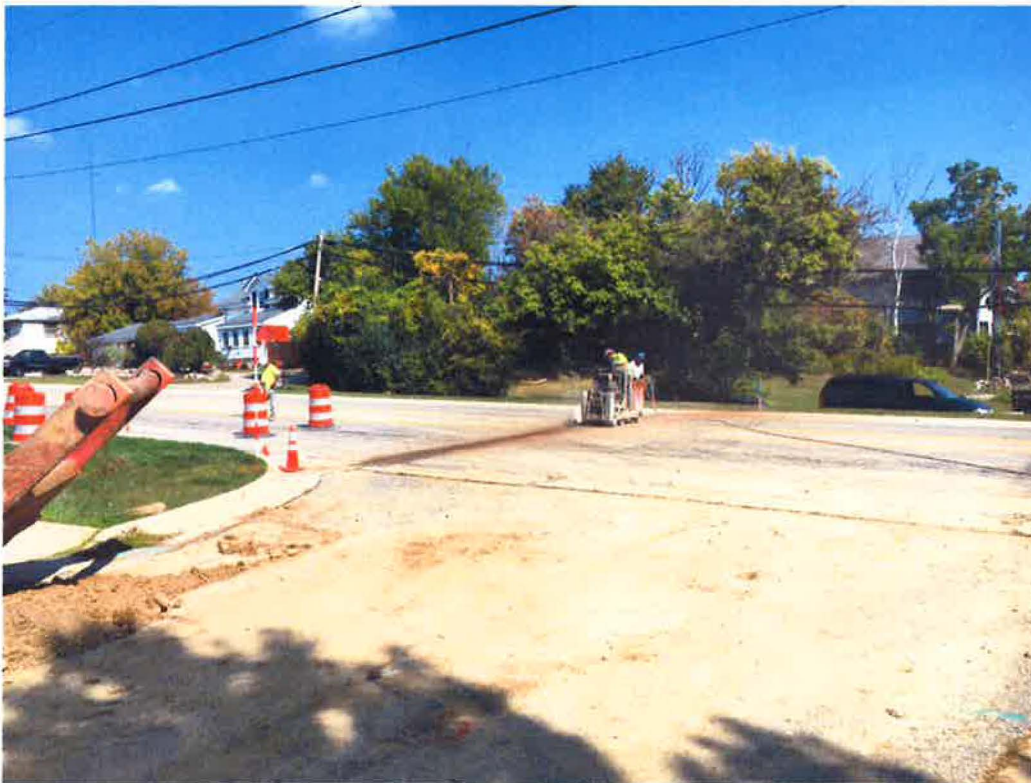
Removing existing asphalt on Taft Road for installation of new water main
