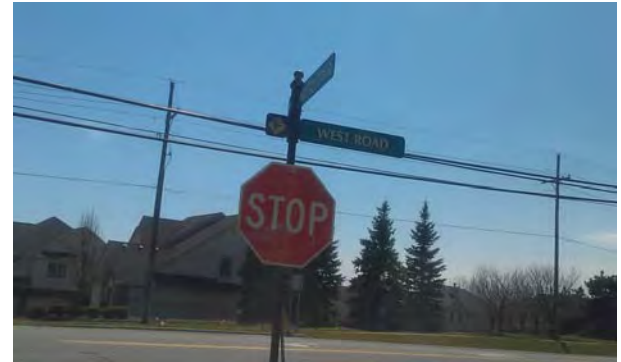
The pole is leaning, the stop sign is faded and the street name sign lettering is peeling and faded. Also, the street name sign should read West Park Drive instead of West Road.
