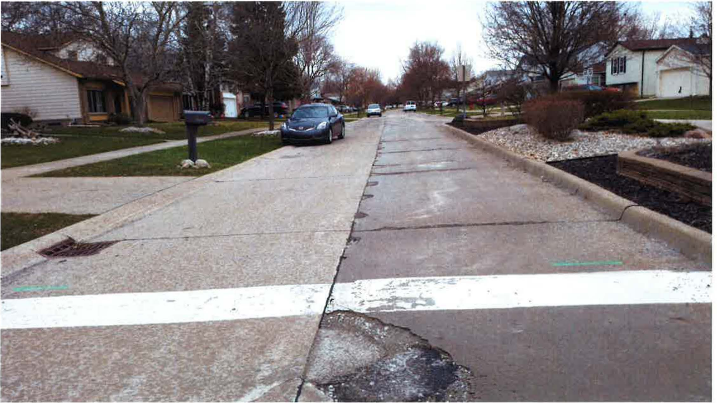
Pre-Construction photo example of the southbound lanes of Kings Pointe Drive boulevard at 10 Mile
