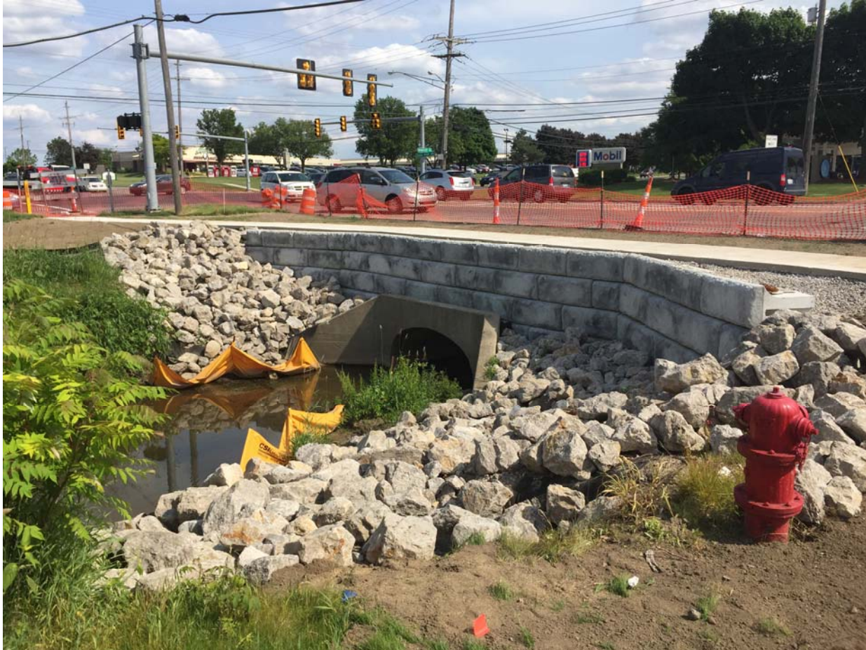
Replacement of existing sidewalk and culvert stabilization: northside of Grand River Avenue, west of Haggerty Road (Mercedes Benz Showroom)
