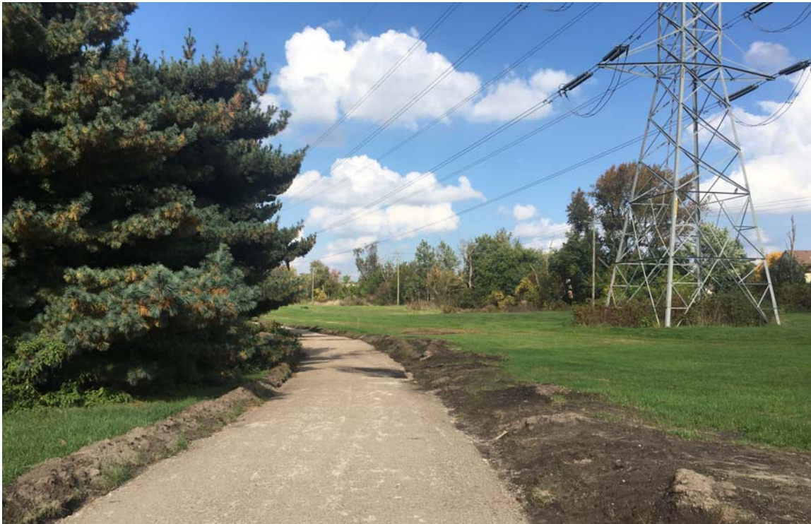
ITC Trail from Nine Mile Road to Eleven Mile Road under construction
