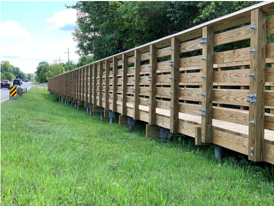
West side of Beck South of Bellagio: New helicals and full replacement
