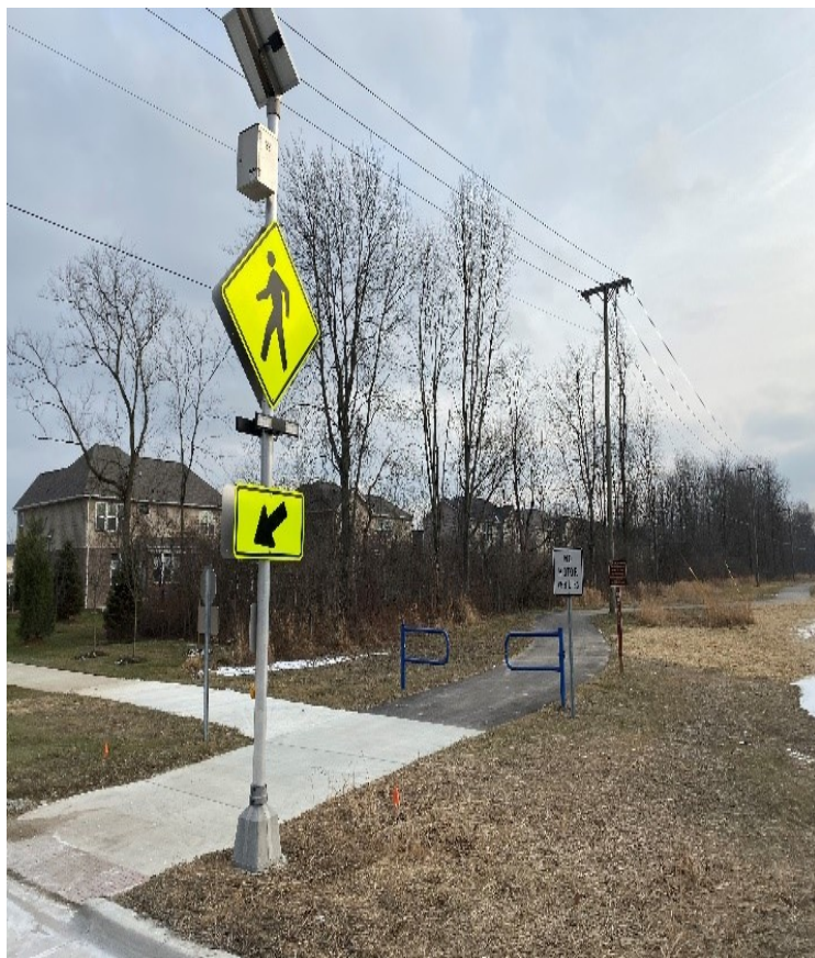
Installation of RRFB's (Rectangular Rapid Flashing Beacon) at the crossings of 10 and 11 Mile
