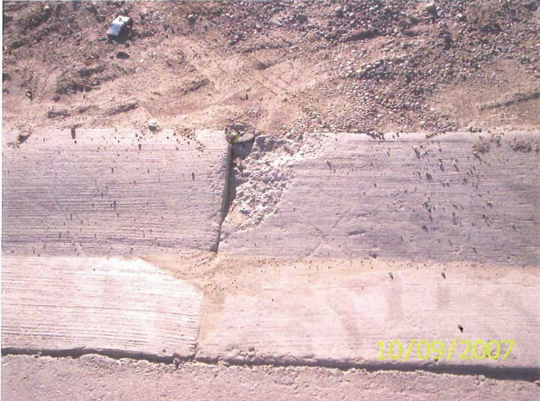
This is a section of curb where the back has been chipped off.
