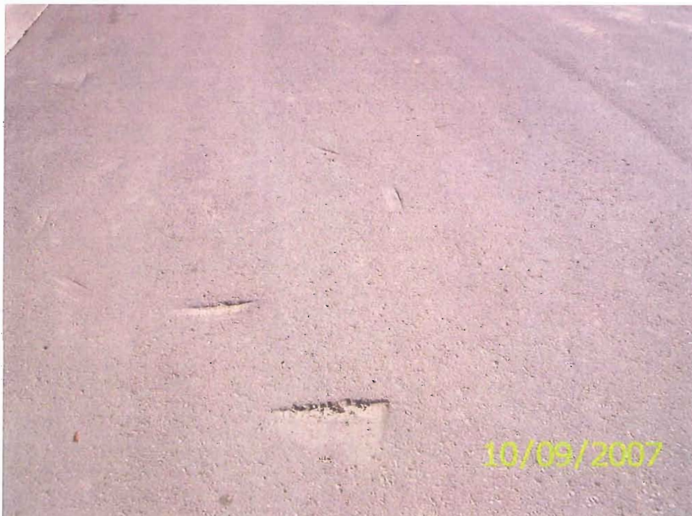
Indentation in the pavement surface could have been a roll off dumpster.
