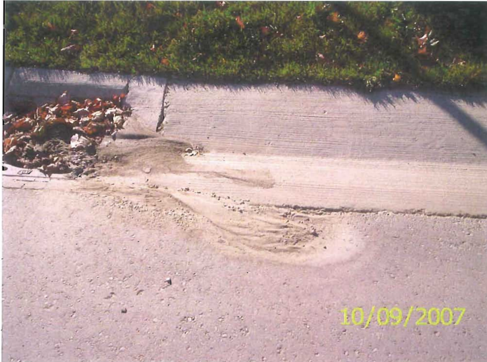
One of the low spots located in the pavement next to the gutter edge.
