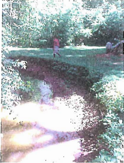
Photo 16: Eroded pool in ROW north of Chattman
