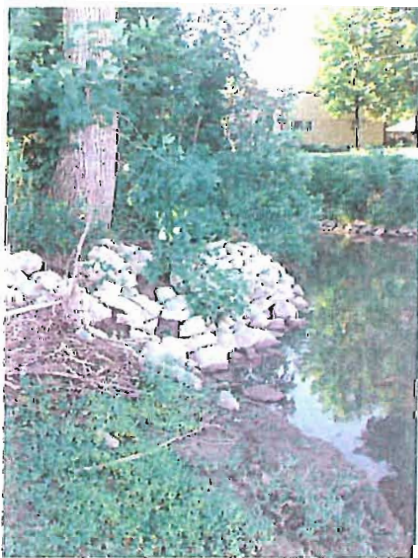
Photo 18: Example of riprap protection (Plumbrook Drain, Sterling Heights, MI)
