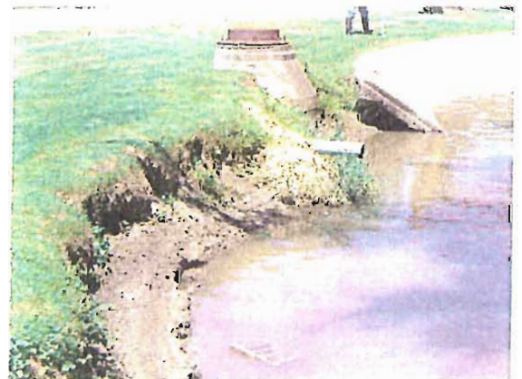
Photo 2: Erosion at outlet of the concrete channel
