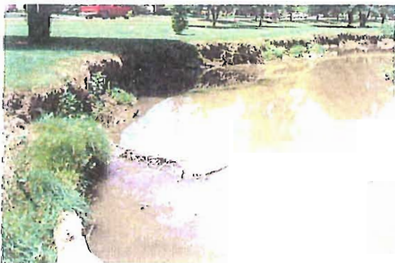
Photo 1: Streambank erosion downstream of Meadowbrook Lake Dam
