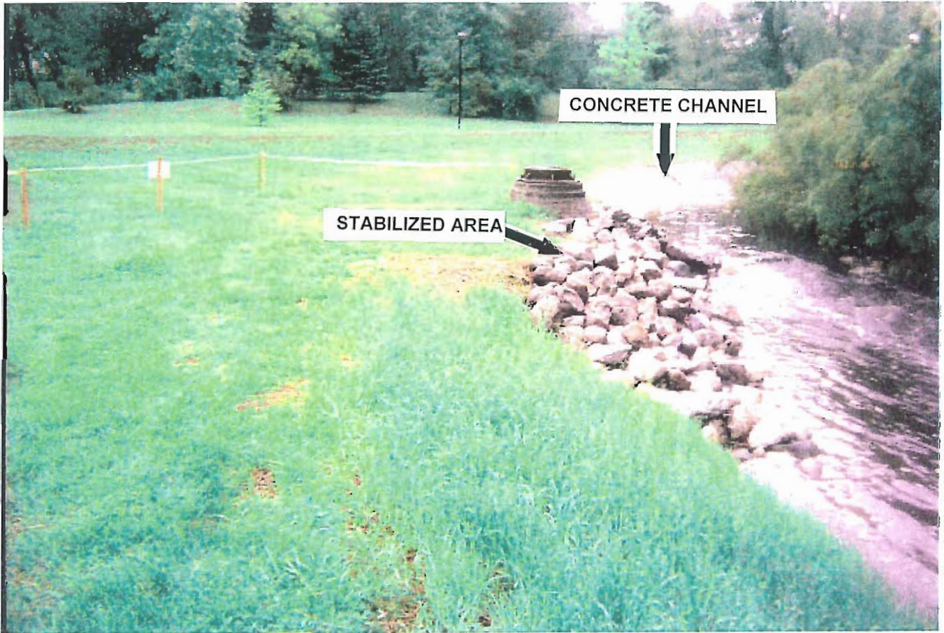
Concrete channel to be removed ( background ) and stabilized area around sanitary manhole ( foreground ).
