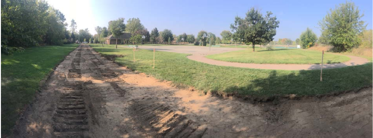
Segment # 4064: Regional pathway connecting the ITC trail at ITC Community sports park to Eightmile road, currently under construction
